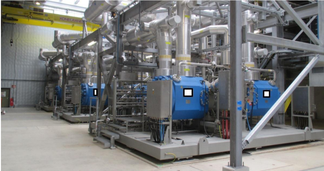
Compressor area where 6 compressors of 12 MW each are located (logo of manufacturer hidden on purpose).
