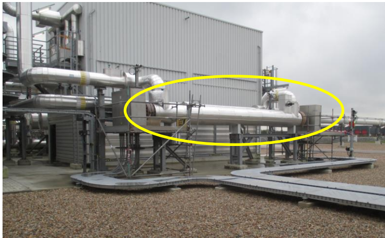
Location of electrical heater bundles
